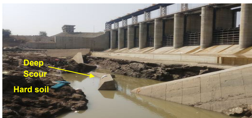
Scour downstream of Balegaon Barrage
