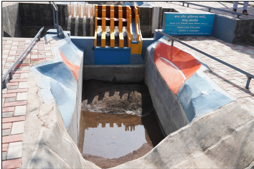
Scour Pattern for Ungated Operation of Spillway for the Discharge of 10534 \text{ m}^3/\text{s} (100%) at RWL El. 1367.5 m
